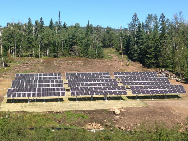
Arrowhead Electric Cooperative, Inc's 40 kW Community Solar and Great River Energy's 20 kW Solar System Lutsen, MN
